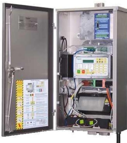
Slika 9: Kontrolna omarica za odklopnik (Vir: U-series. Pole mounted Auto reclosers overhead distribution network, 2018)
